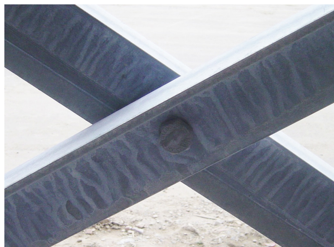
Fig 1. Wet storage stain formed on galvanized surface
