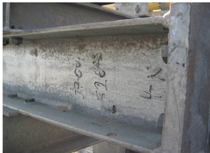
Fig 2. Uncoated areas due to paint markings not removed prior to galvanizing
