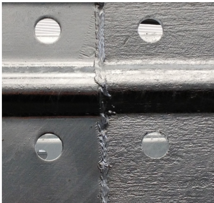
Fig 3. Variation in coating smoothness due to different surface steel chemistries
